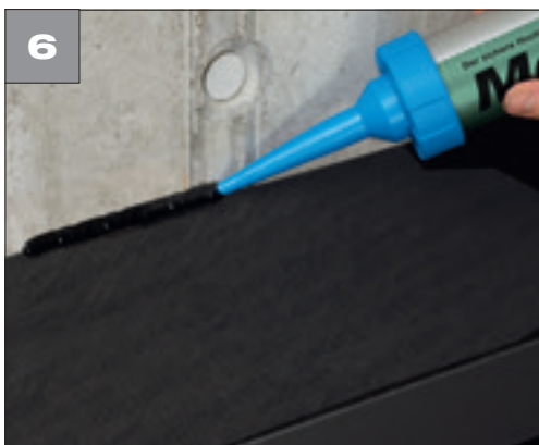
• Fentes, joints, imperfections
